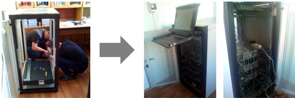
Fig. 3. Process of the cyber range hardware installation
